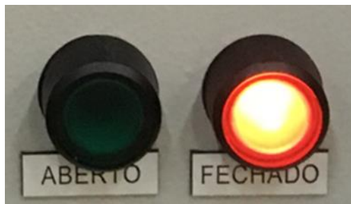
Figure 19 – Recommended solution for the pushbuttons and LED signalization of the actual position. Not represented in the figure, also a visual indication of the Local control status is mandatory.
